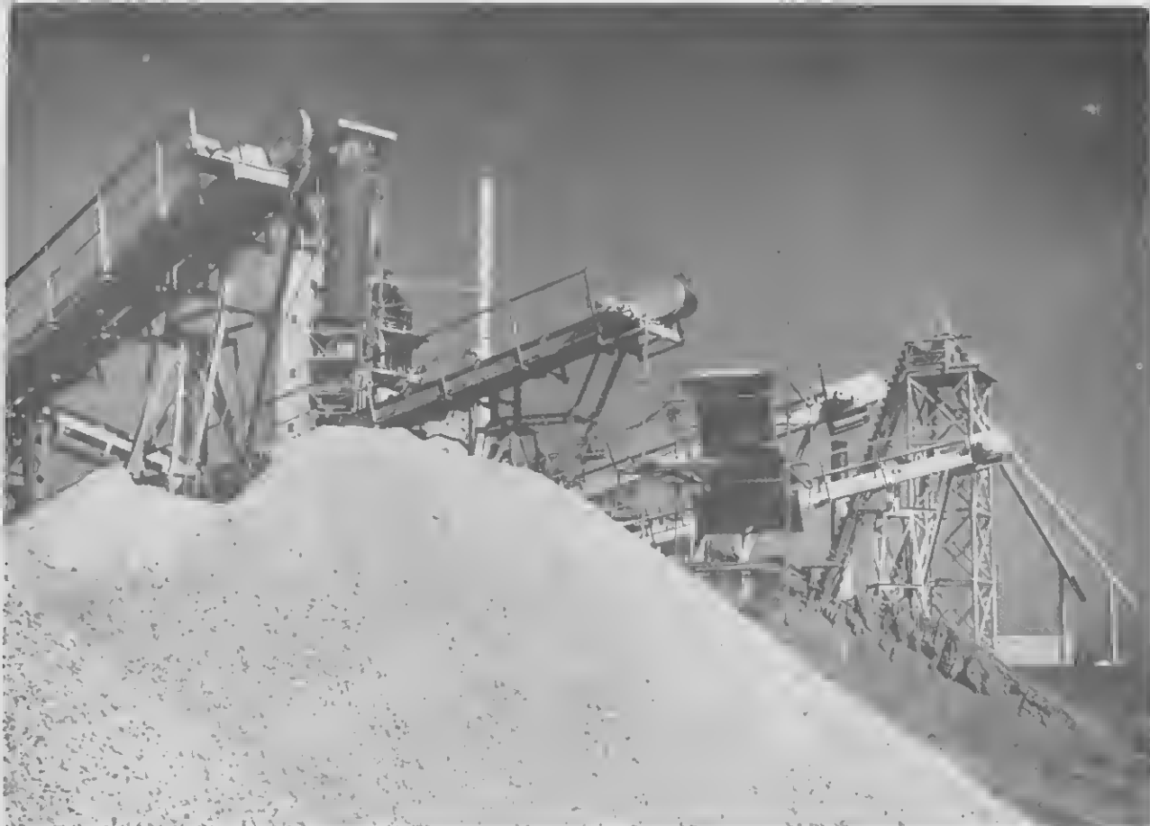
ROCK AND sand pile up on the seaward side of the Concrete Plant. The conveyors drop fresh stocks on the pile as needed, and just incidentally form interesting patterns against the sky for the photographer.
